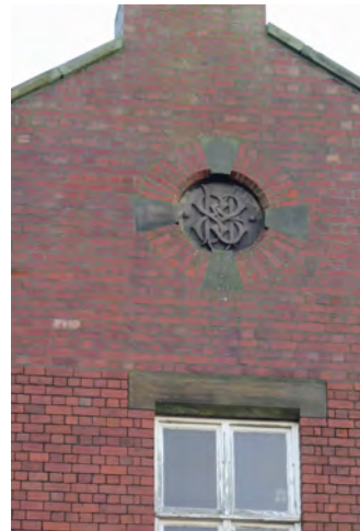
Fig.243 Inappropriate cement pointing
