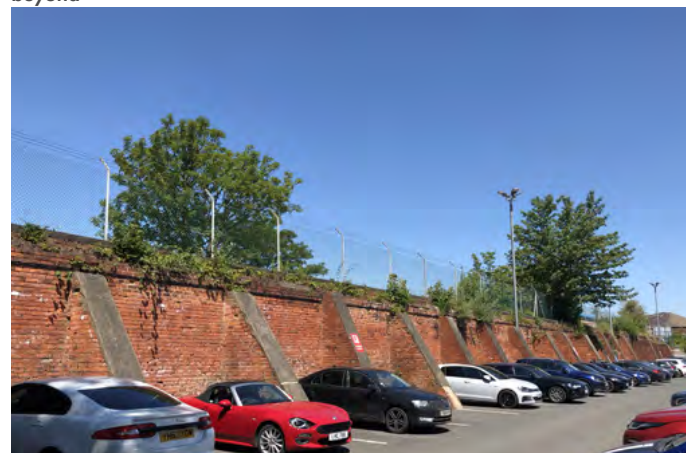
Fig.266 Coal drops with the original coal cells trimmed back to form buttresses
