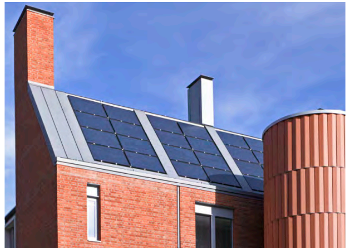
Fig.331 Example of solar roof panels integrated into the roofscape, flush with the roof covering ✓
